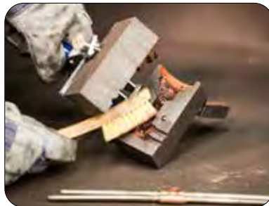
Step 7: After the connection is complete, open the mold and remove the connection, remove slag and clean mold before making the next connection.
